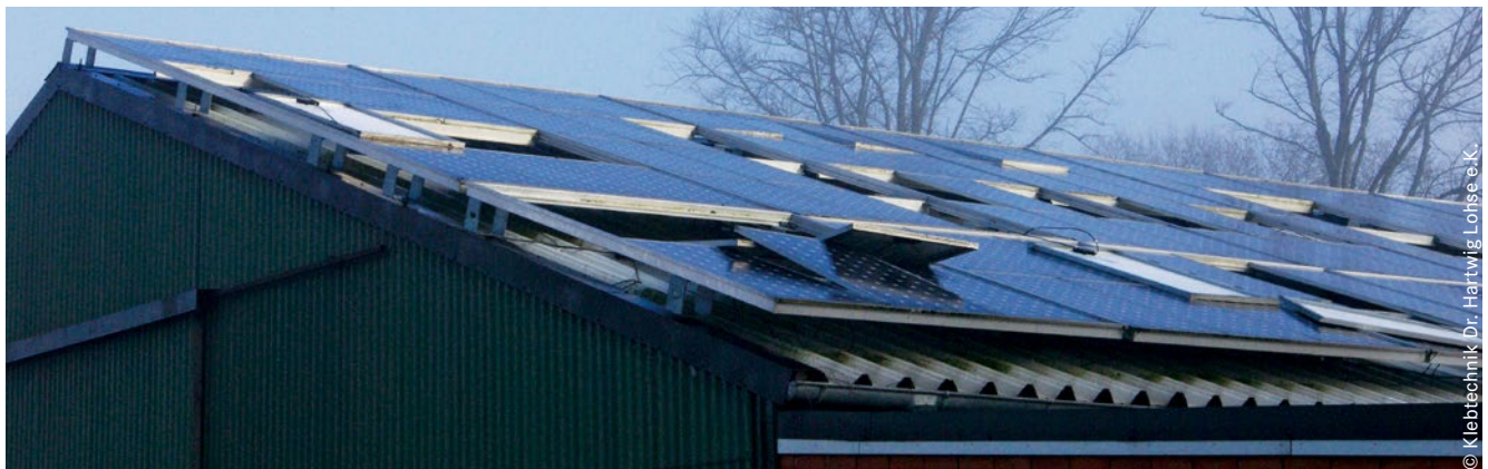
Figure 1: Row by row failure of bonded joints after exposure to high winds. Joint failure between the solar modules and aluminum base due to serious bonding faults
